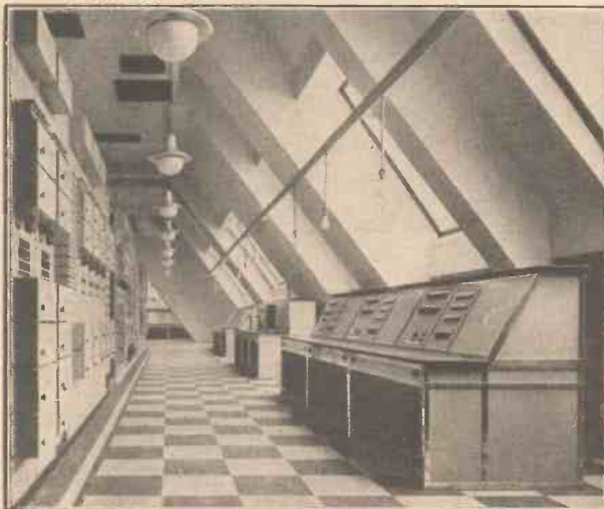
The magnificent new control room, under the eaves of Broadcasting House, provides for the balancing of every programme—whether from studio or from outside—before it is forwarded to the transmitter.
