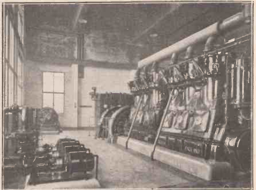
A corner of the Skithwaite Power House, showing one of the four 345-horse-power Diesel engines.
