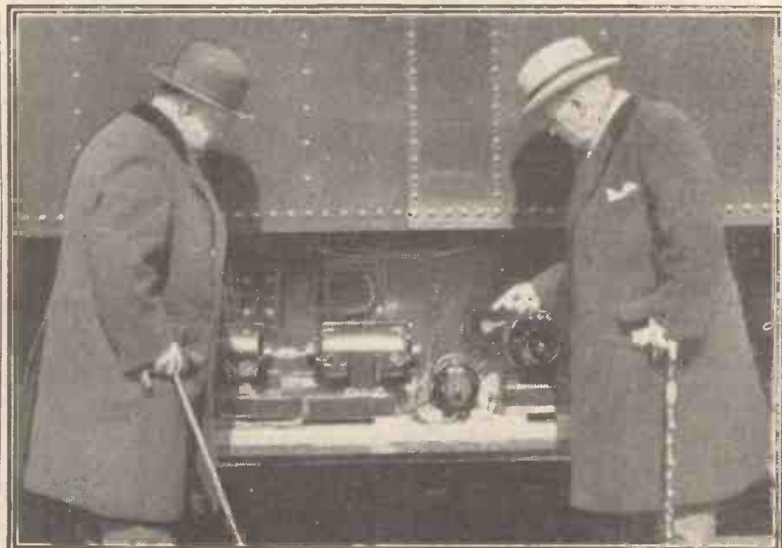
The generators and main apparatus for the railway telephone system is mounted below one of the cars, and can be seen in this picture.
