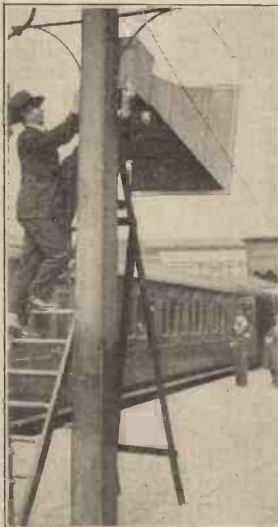
Fitting one of the large loud speakers on London Bridge Station to be used for crowd control during the rush hours.
