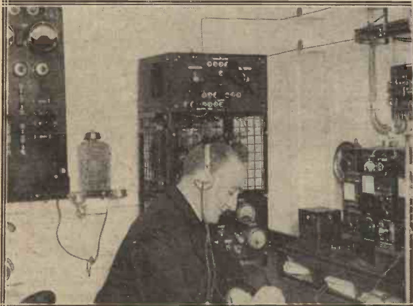
Although telephony is used to some extent on the larger liners, Morse is still the main means of communication. This is the elaborate installation on board the motor liner "Alcantara," where a special system is provided to enable the Daventry programmes to be distributed all over the ship when desired.
