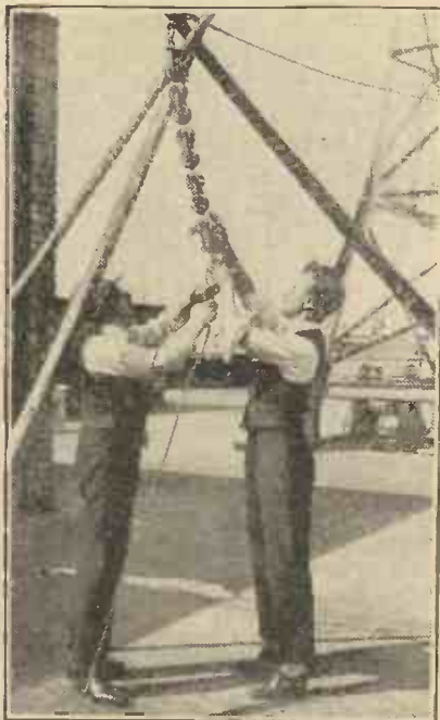
Cleaning the insulators of the aerial at the London station—a regular and necessary practice.
