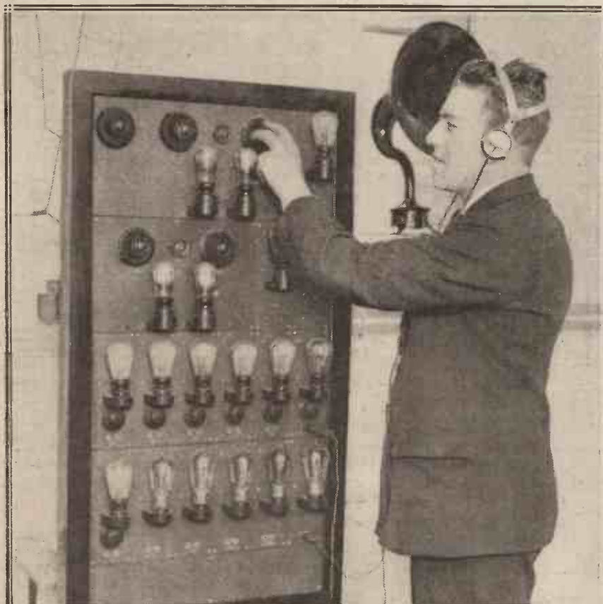
Making adjustments on the nineteen-valve receiver and amplifier installed in the Lambeth Hospital. It supplies 2,000 headphones and 80 loud speakers with either broadcasting or electrically reproduced gramophone records.
