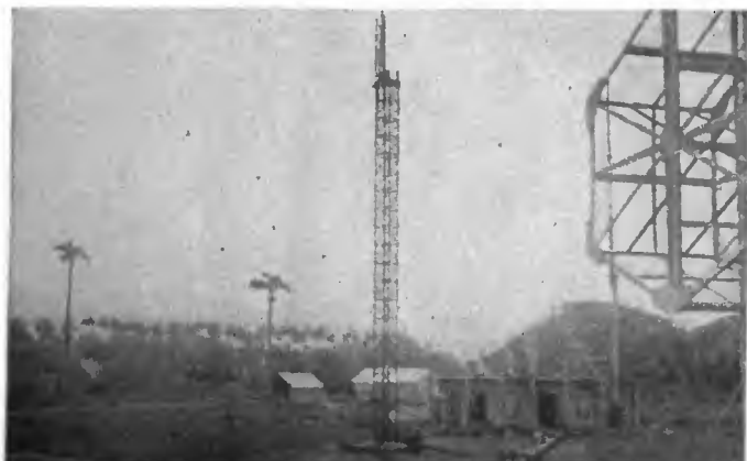
Going up—the central mast for the radio station at Cayenne, French Guiana. At the right is a portion of the big loop used for receiving
