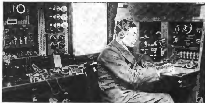
A corner of the operating room of the Radio Corporation of America showing some of the control instruments
