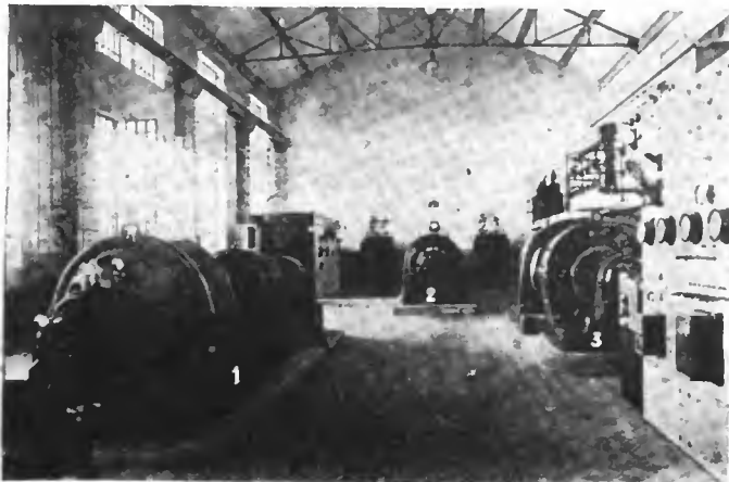
Figure 4—At the back, the spark sets and the transformers. In the foreground, the Bethenod Set. To the right, the 3-phase motor-generator set driving the H.F. set
