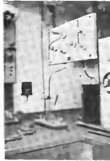
Loading coil panel and antenna switch
