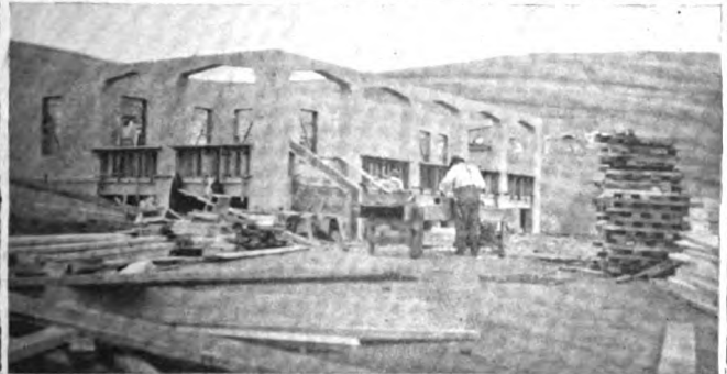
Completing the first floor of the Assistant Engineer's Cottage at Marshall's, a fine type of the Modern fireproof bungalow.
