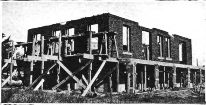
The Operating Building at New Brunswick, where all the Edifices combine sightliness with utility
