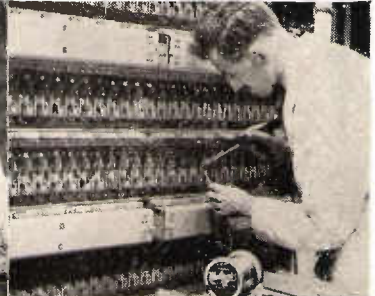
TELEPHONES Automatic Exchanges each having more than a million soldered joints; are made to last a lifetime with ERSIN MULTICORE SOLDER.
