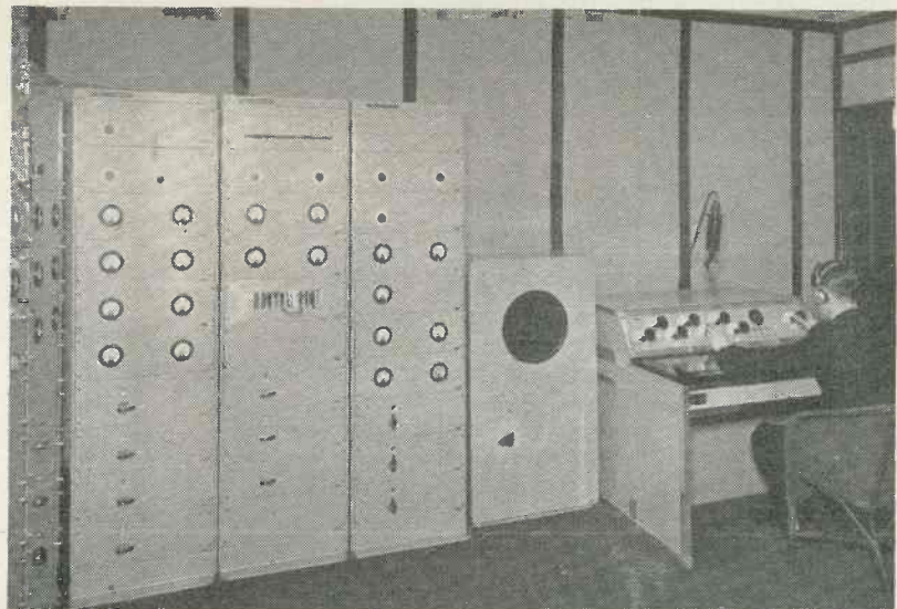
The Baird control panels for the Alexandra Palace.
