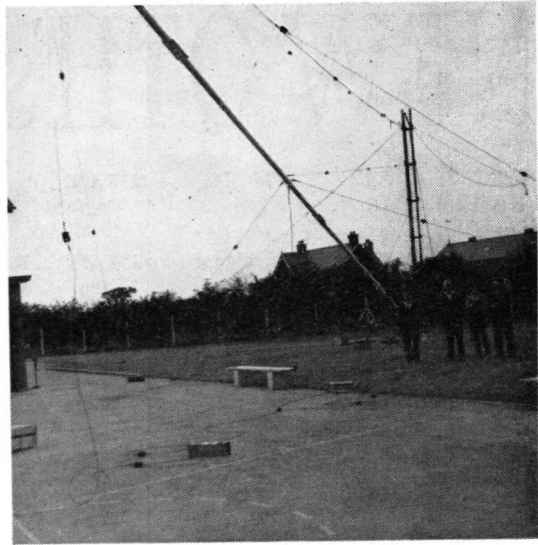
The Rawstorne School 86-ft. mast going up, with the staff responsible for the erection. Raising was by a 25ft. boom, and hauling by block-and-tackle, and took about five hours of agonisingly slow movement; the guys had to be adjusted by car headlamps, as the light had gone by the time the mast was in the vertical. Since its erection, the mast (which has become a local landmark in the Croston district of Lancashire) has withstood severe gales without a tremor. (See p.259, July and p.329 this issue).
