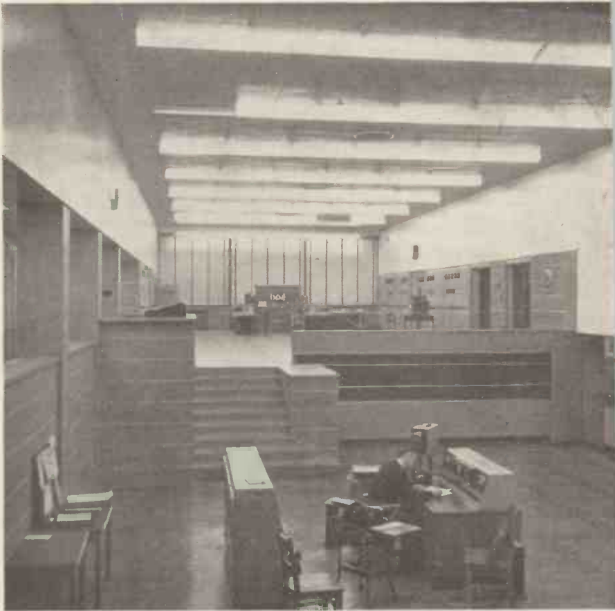
General view of the Canadian Broadcasting Corporation's International Service transmitter hall at Sackville, New Brunswick. The transmitters themselves are ranged round the walls on the upper level and are controlled from the operating console in the foreground.
