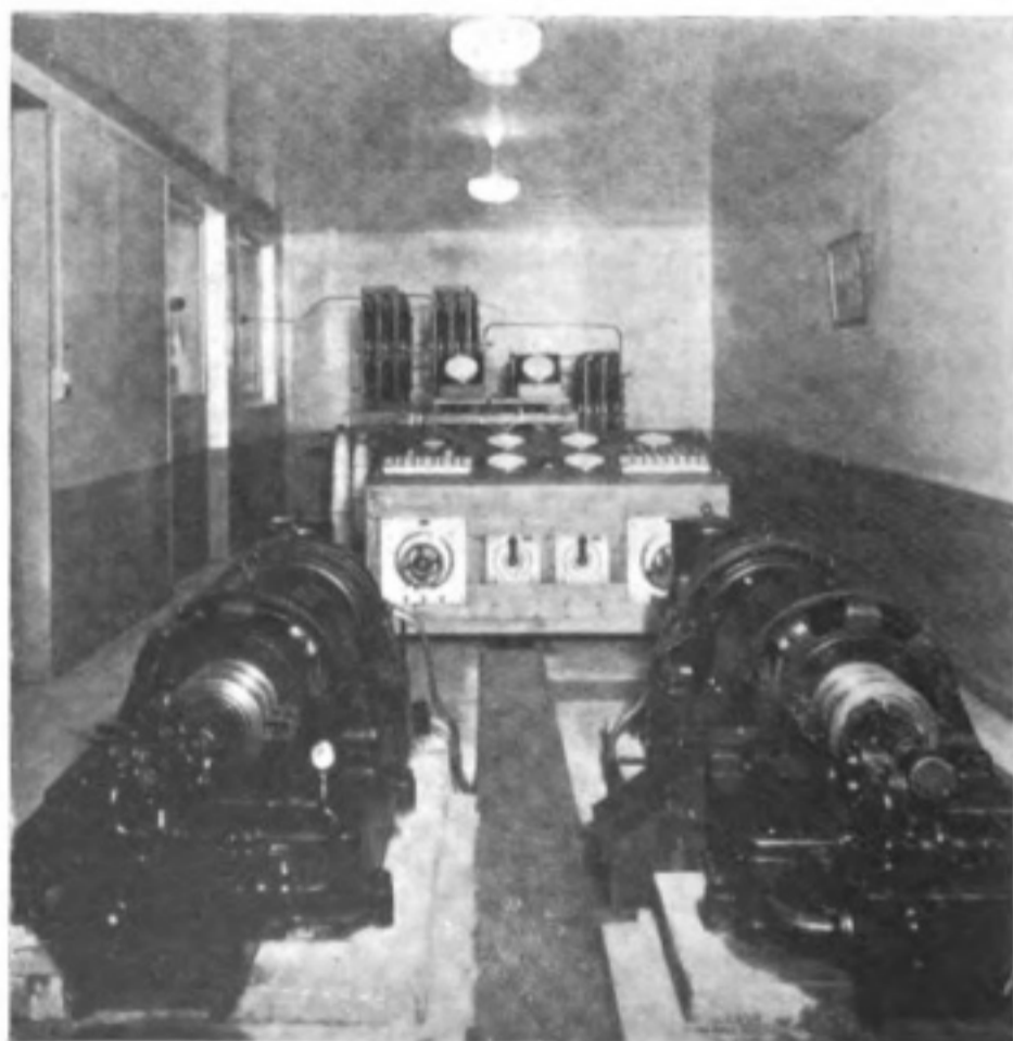
FIG. 2.—50-kW Transmitting Installation at the Levallois Works.
