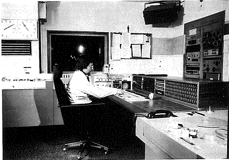
Herr Mausbacher at the automatic controls in the network room, Cologne, Germany.
