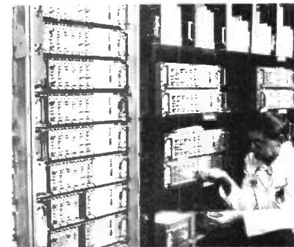
Base station equipment
