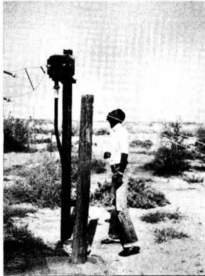
A communications technician in Mauritania (5T5-land) examines a 1kW balun unit that is connected between the 50Ω coaxial cable (seen coming out of the ground) and the feed-line on the log-periodic antenna
