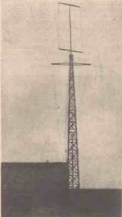
New aerial system installed at the International Short-wave Club (London Chapter), R.A.C.S. Hall, Wandsworth Road, S.W.8. Provision is made for television, also for short-wave transmission and reception. The television feeder comprises some hundred feet of Telcon A.S.S.C. cable.
