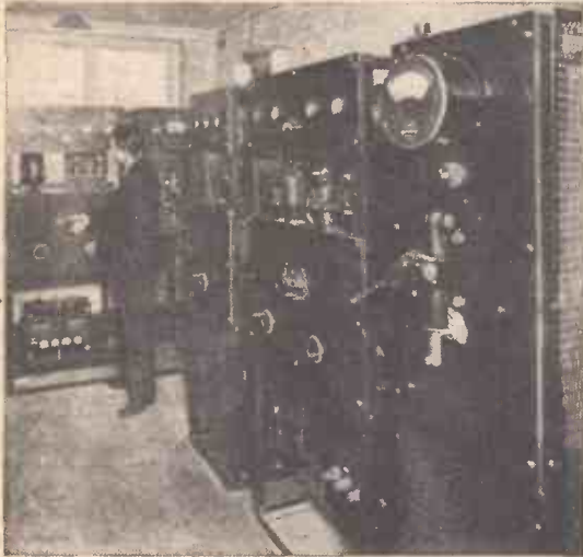
Fig. 1.—A view of the amplifiers and control panels of a modern transmitter.
