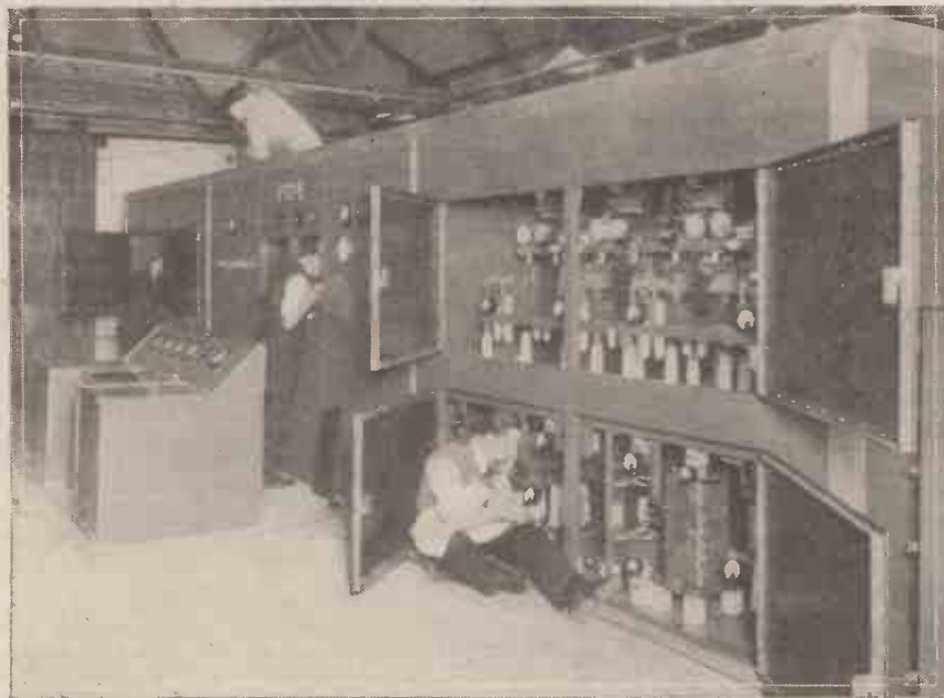
The transmitting equipment for the new broadcasting station to be erected by the Government of Palestine is now nearing completion at the Marconi Works, Chelmsford, and this photograph shows fitters at work preparing the transmitter for its final tests before packing and despatch. The three main panels of the transmitter are shown, together with the control desk. The power of the station will be 20 kilowatts unmodulated aerial energy, and it is to be erected on a site about seven miles north of Jerusalem.
