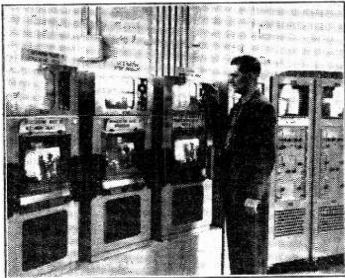
Part of the Monitoring Bay at the G.P.O. Switching Centre in London.
