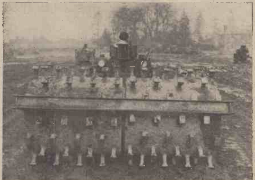
A "sheepfoot" roller for pummeling the ground, being pulled by a bulldozer. These specially formed rollers will be largely used after the war for housing clearance and road construction.
