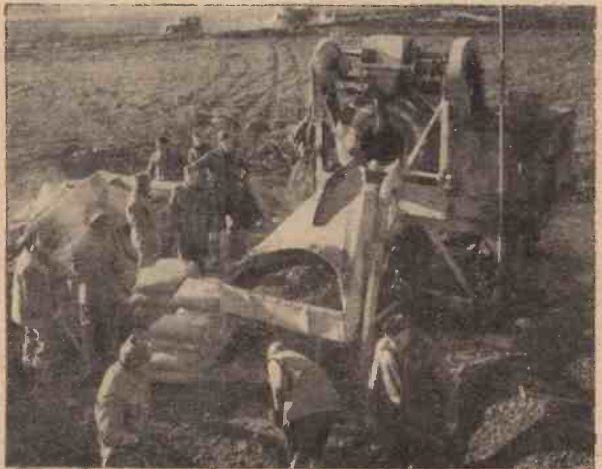
Into the mixer the men shovel sand, stone and cement, which will transform the mud into a flat concrete stretch.
