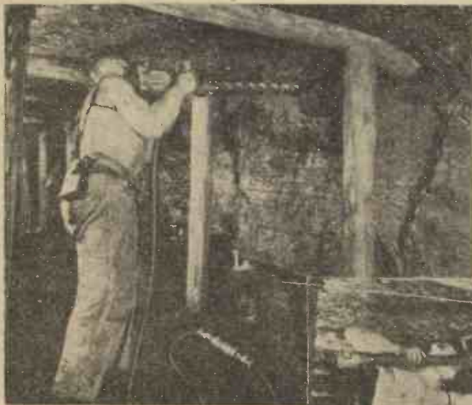
Fig. 1.—(Above) Drilling the coal ready for insertion of the burster. Note that the coal is already undercut and is supported. Fig. 2.—(Right) Inserting the burster.
