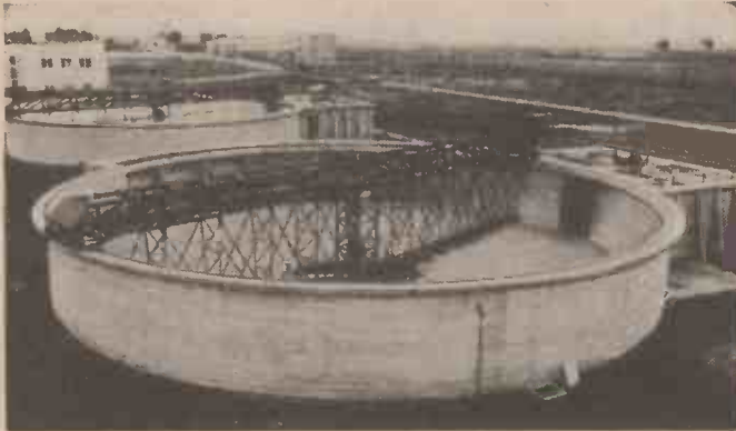
Clarifiers as built at Siouf, Alexandria
