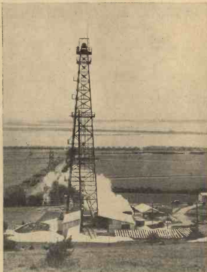
The first large-scale attempt to discover whether Britain contains sufficient oil to satisfy her needs and to free her from almost total dependence on foreign supplies was inaugurated recently on Portsdown Hill, above Portsmouth Harbour, where drilling operations were begun. The plant is capable of driving a 2-ft. diameter bore to a depth of 3 miles, and the huge derrick 136 ft. high, forms a new landmark on the horizon.
