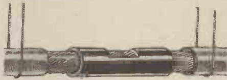
Fig. 4.—When soldering two wires together, an efficient joint can be made by using sleeving over the two ends as shown.
