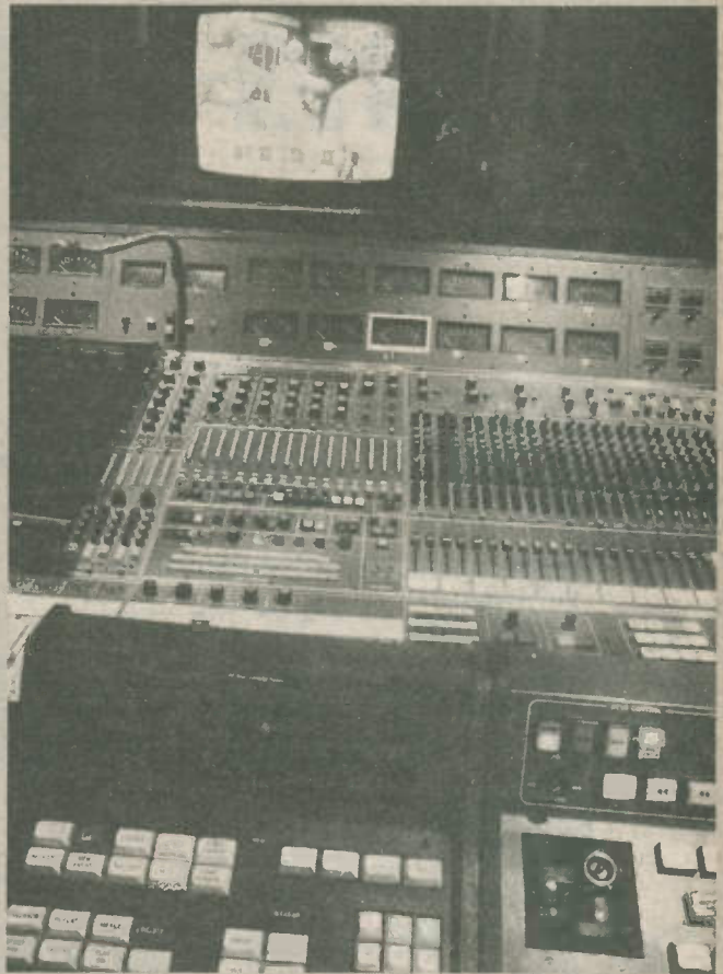
Control desk with time code visible on monitor screen
