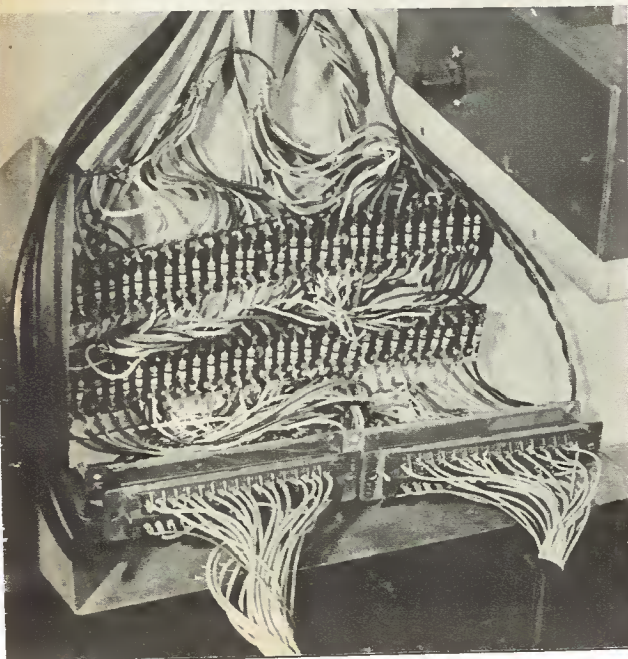
Pedal resistor boards in position on console kneeboard. Here the pedal plugs are shown mated to the sockets
