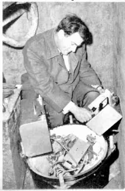
An underground repeater on the p.c.m. link between Reading, Maidenhead, and Slough
