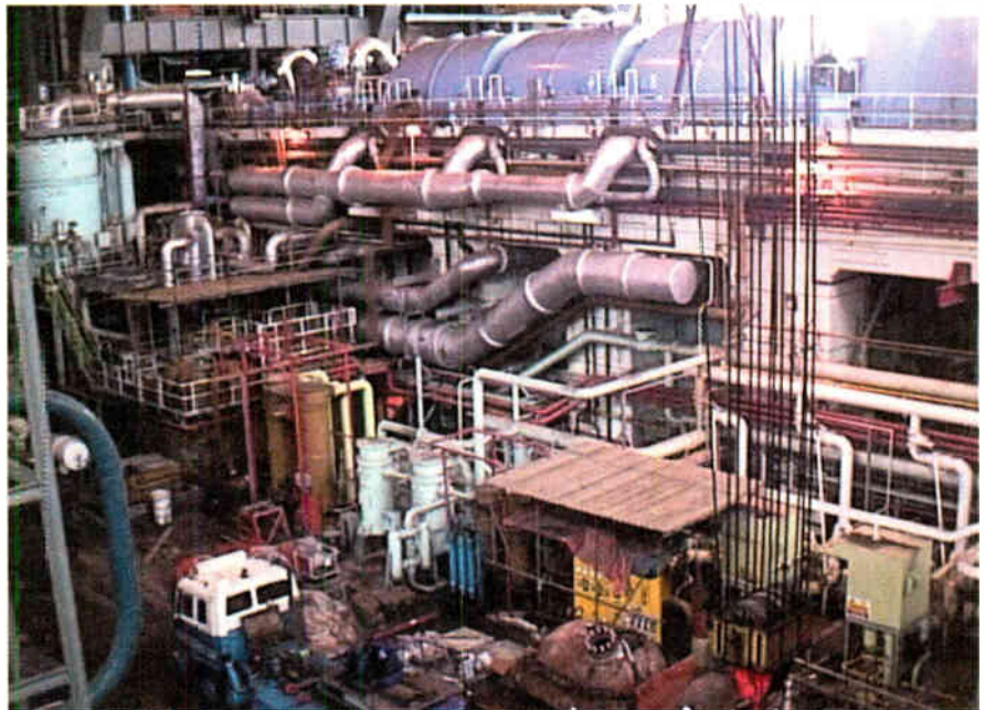
The generator hall at Ironbridge, showing one of the two turbines and generators.
