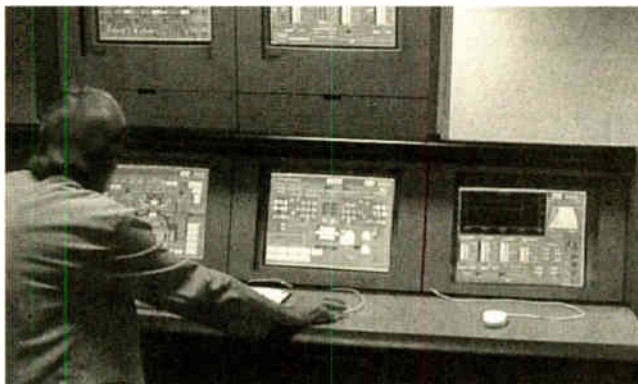
At the control desk, the operator uses a mouse to control the power station.
