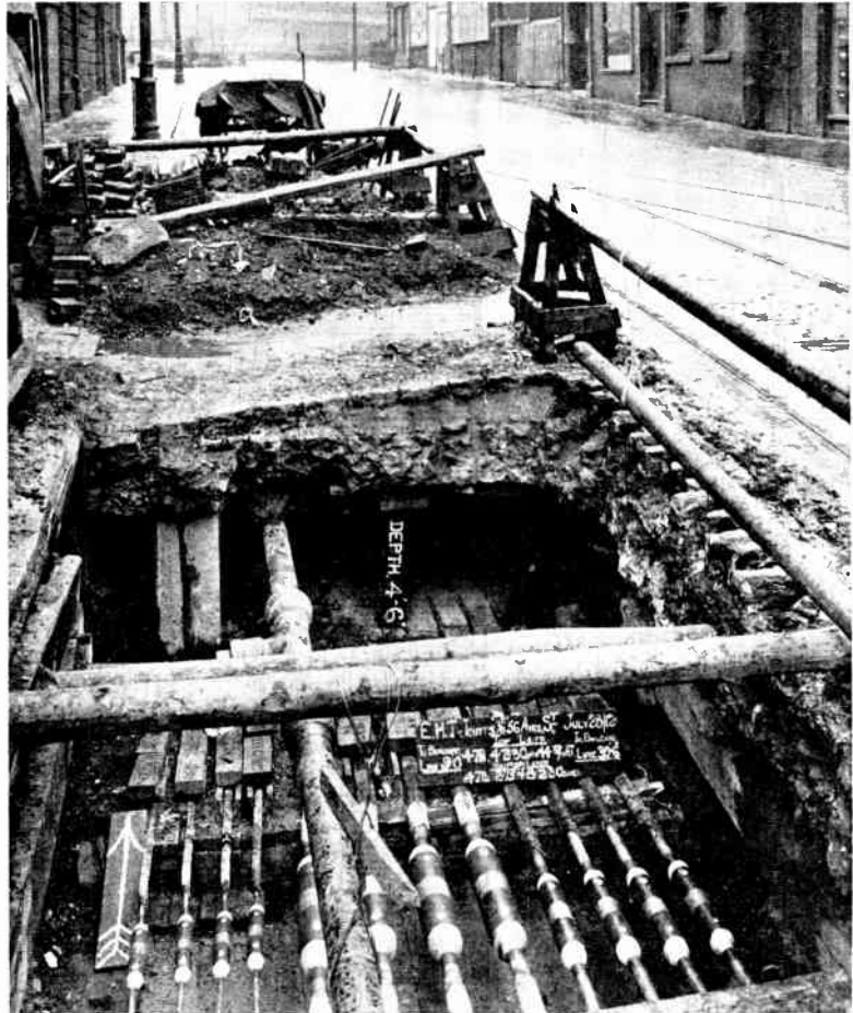
Fig. 26.—ANOTHER VIEW SHOWING THE LAYING OF H.T. UNDERGROUND CABLES IN CONDUITS. (W. T. Henley's Telegraph Works, Co., Ltd.)
