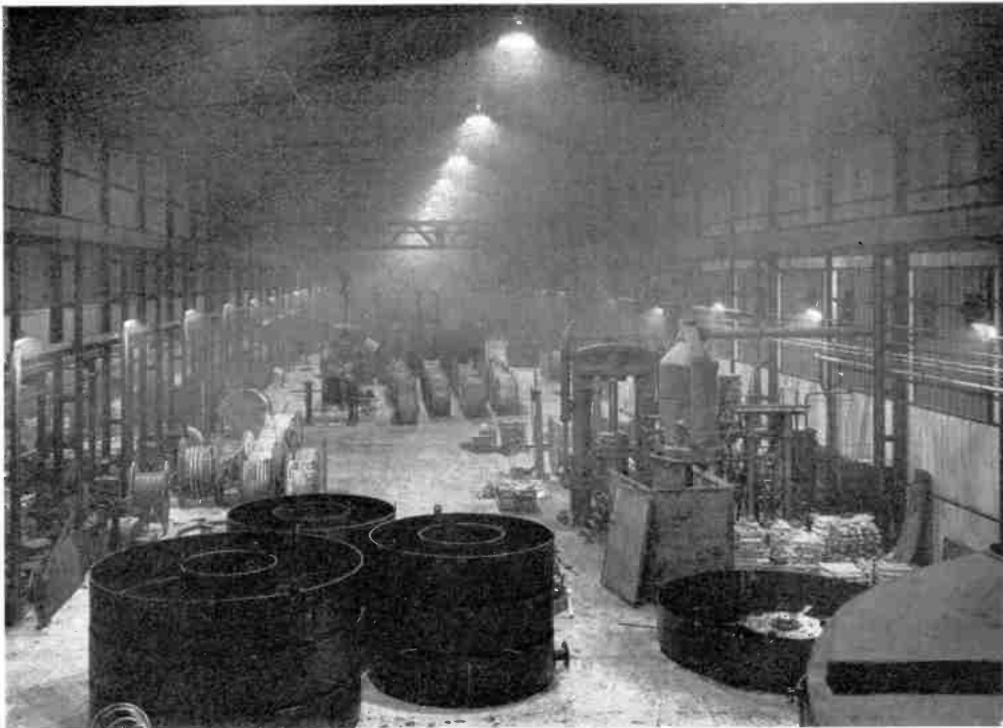
Fig. 6. —LIGHTING SCHEME FOR LARGE FACTORY WITH CENTRAL LIGHTS ABOVE CRANE. (E.L.M.A.) In this case the central lighting has been supplemented by brackets fitted to the side stanchions to give additional general lighting.
