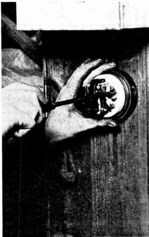
Fig. 1. —FITTING A DIMMING SWITCH. Showing how a 60 watt dimmer switch can be substituted for a 5 amp. tumbler switch on the same 3\frac{1}{2} -in. switch block.
