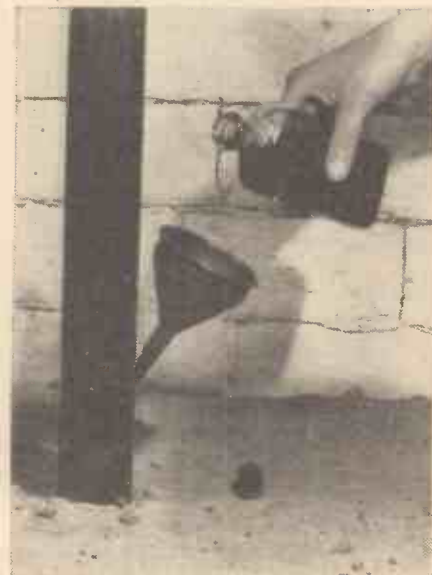
The creosote is poured into the hole in the base of the mast at intervals of a month or six weeks.
