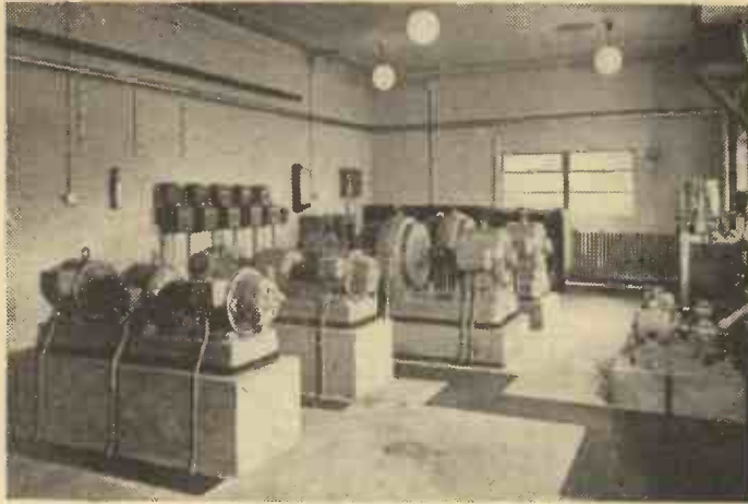
The filament and G.B. generators in the machine-room at Penmon, Anglesey. Both machines are duplicated in case of breakdown. On the right are pumps for water cooling the anodes of the transmitting valves.
