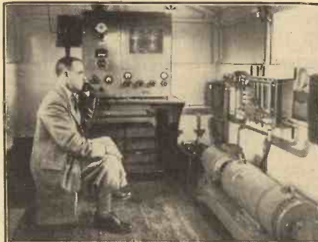
Owing to the growth of air-liner traffic in the south and west of England, the Air Ministry recently decided to install a mobile radio station at Portsmouth pending the construction of a permanent station. This photograph gives a glimpse of some of the apparatus inside the special mobile unit, one of the duties of which is to keep in touch with mail planes catapulted off transatlantic liners.
