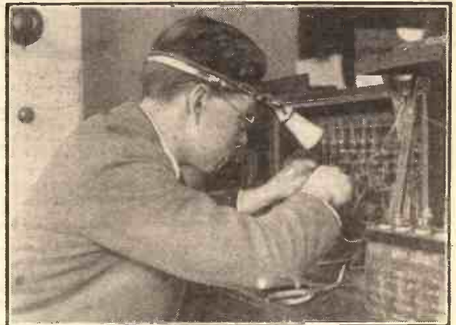
Behind the control panels at Broadcasting House there is an intricate mass of wiring which often requires examination. The engineer employs an ingenious inspection lamp, which keeps both hands free.
