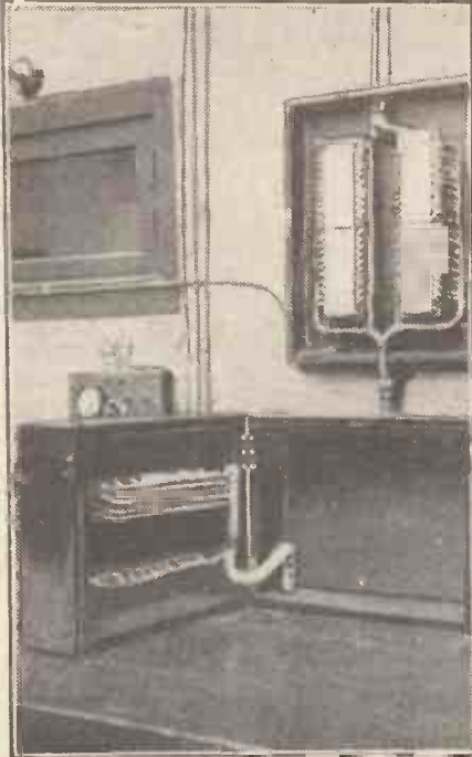
Junction and switch-board boxes where hundreds of telephone lines terminate in 2 B E's control room. All this wiring was carried out by the station engineers, and is remarkably neat.
