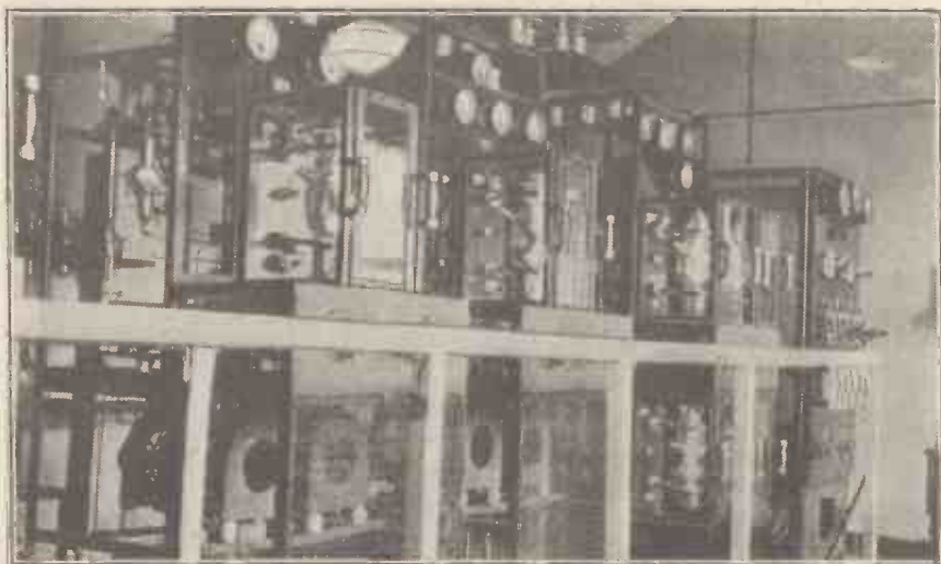
The transmitter at 2 B E. It is a standard outfit and is installed at the Corporation Power Station in East Brige Street.
