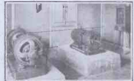
A corner of the generator-room at the Hilversum broadcasting station.
