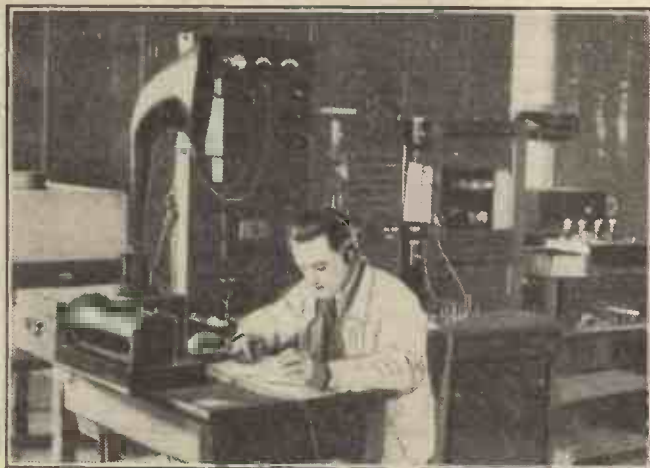
The control room of the Ecole Supérieure, Paris, Station, showing the switchboard which is connected to the various theatres and educational centres.
