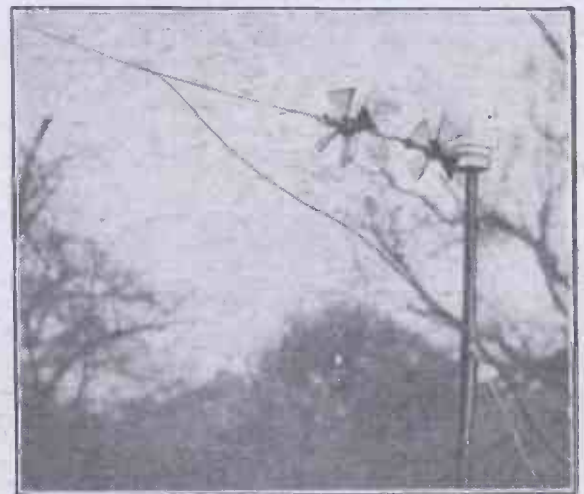
Two of the "Winsulators" fitted to the aerial erected on the roof of Mr. Ramsay MacDonald's house at Hampstead.
