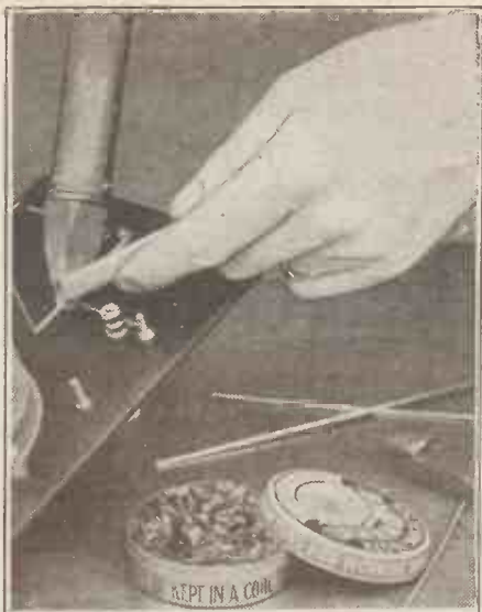
A quick application of a hot iron and solder to a clean joint will result in an efficient connection.
