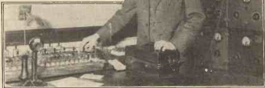
The remote control switchboard in the control room of W J Z, the New York broadcasting station.
