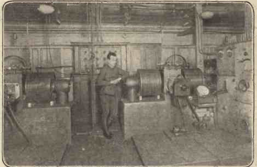
Every amateur is familiar with the signals from Eiffel Tower. This photograph shows the interior of one of the power rooms and the arc generator.
