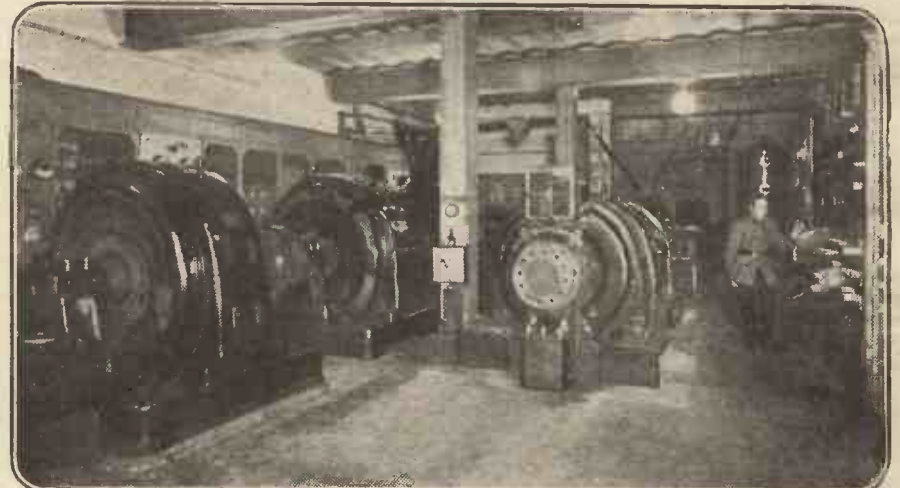
Here are some of the monsters that generate the power at the Eiffel Tower station. A rotary spark gap can be seen on one of the alternator shafts. "Spark" transmissions on 2,600 metres from F L are quite frequent.
