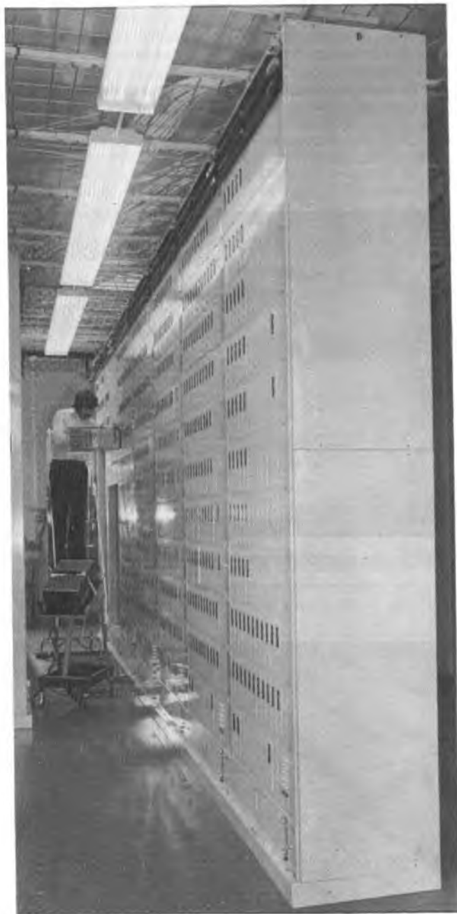
Fig. 6—The Werrington Pentex ERM installation
