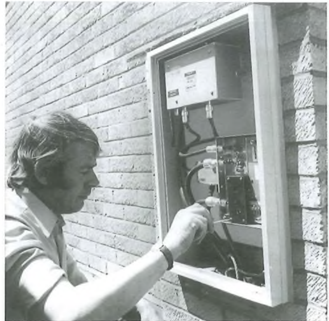
FIG. 3—First-generation VHF-UHF amplifiers in wall box at customer's premises
