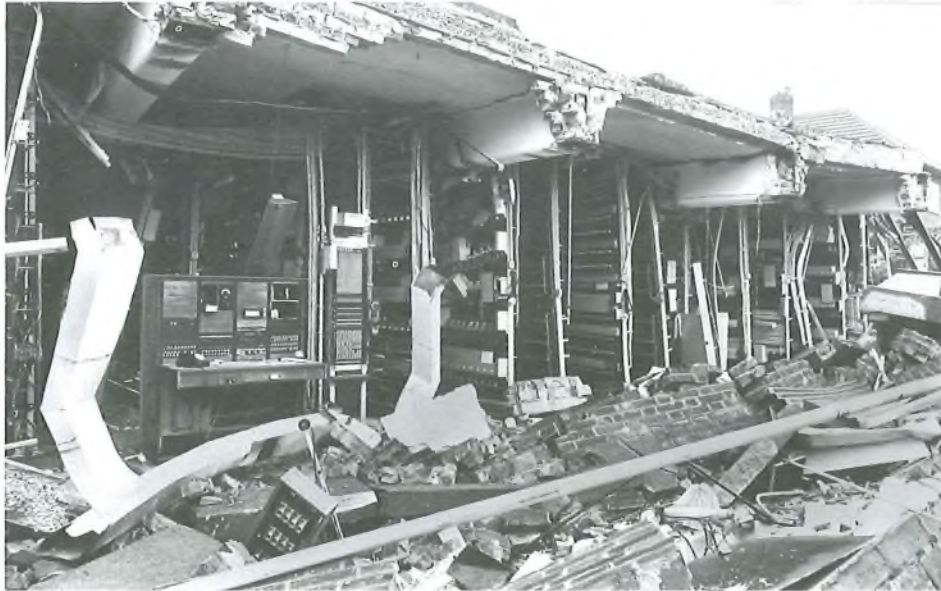
FIG. 2—Bishopwearmouth exchange after gas explosion
