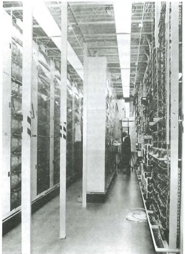
Part of the equipment area at Redhill Clarendon
