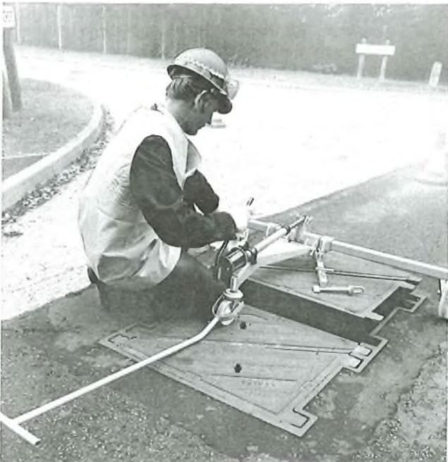
FIG. 1—Use of Lifters, Manhole-Cover No. 4 saves back injuries
