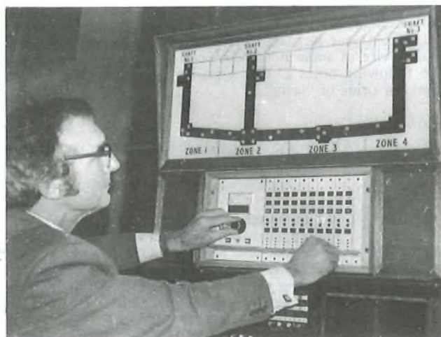
Alarm-indicating and gas-monitoring panels (By courtesy of Becorit (Great Britain) Ltd.)
