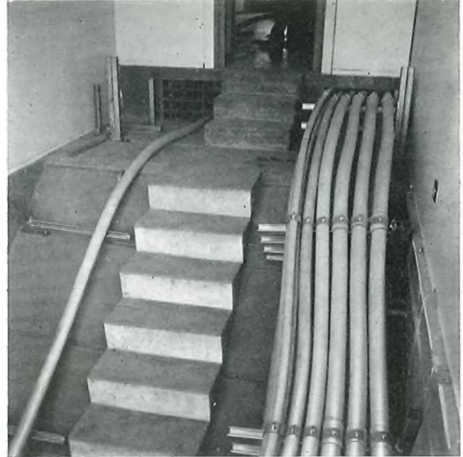
FIG. 4—M-type cable pit showing cable slope and access under the raised floor in the m.d.f. room
