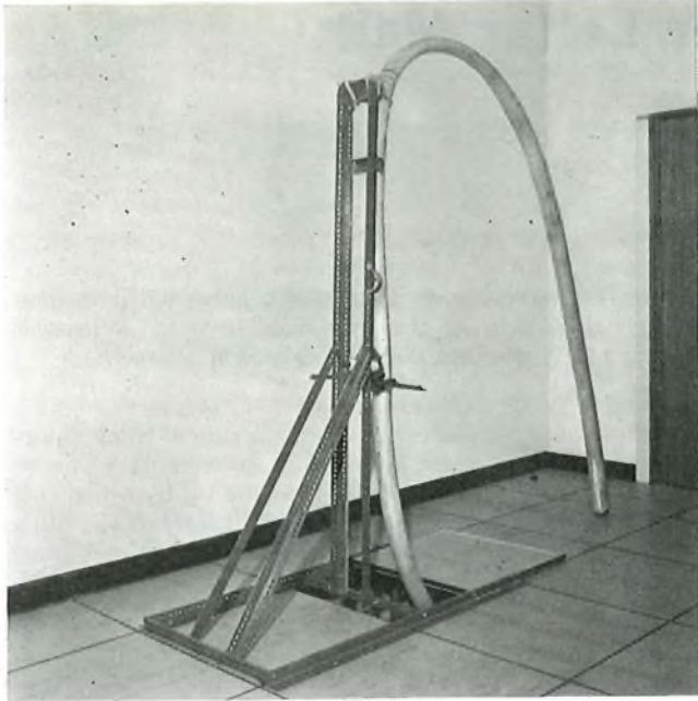
FIG. 5—A 4,800-pair cable in position on temporary rack prior to stripping and making air-block
